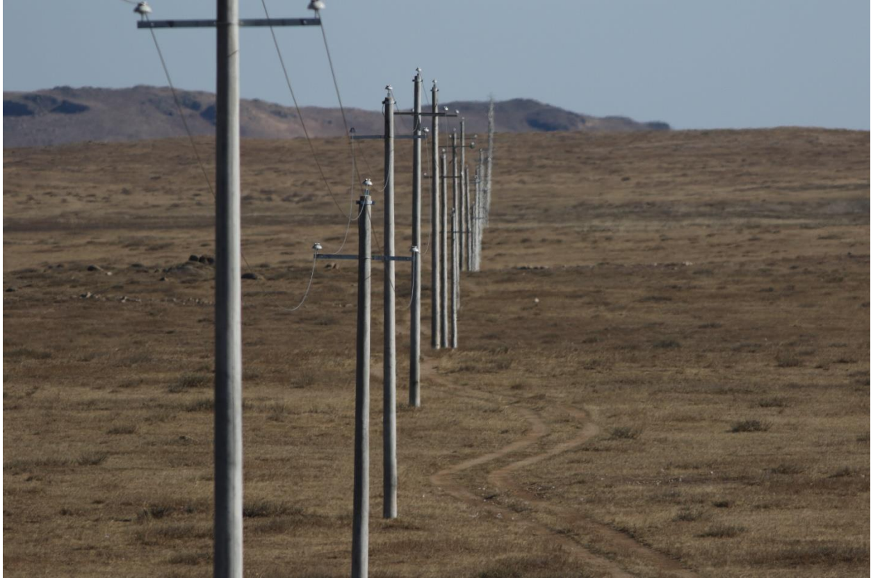
Figure 3. 15 Kv electricity distribution line between Munkhkhan and Uulbayan Villages. Photo taken in 15 th of October.
