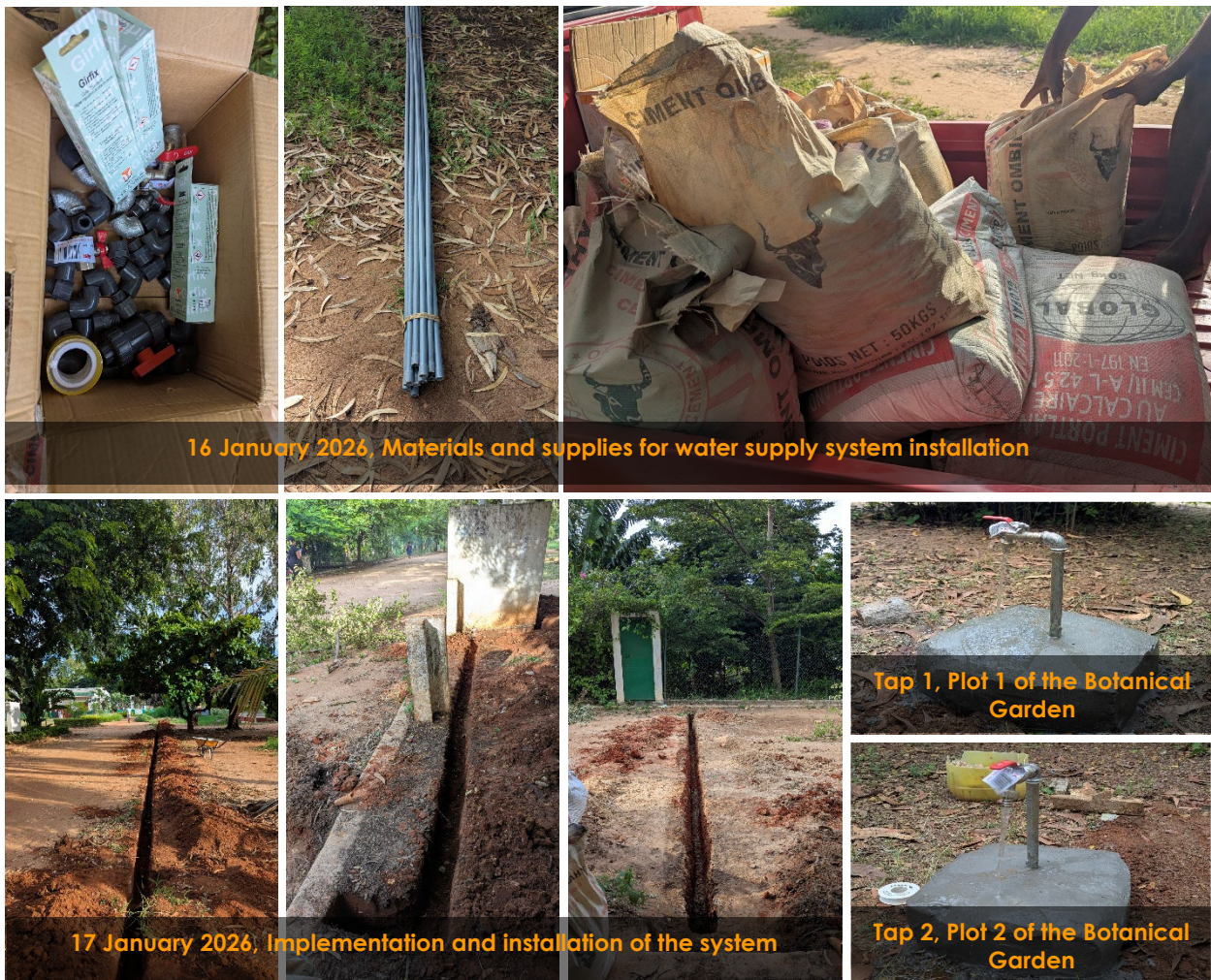
Photo 6 : Water supply system installation enhancing irrigation capacity and ensuring continuous water availability across both plots
