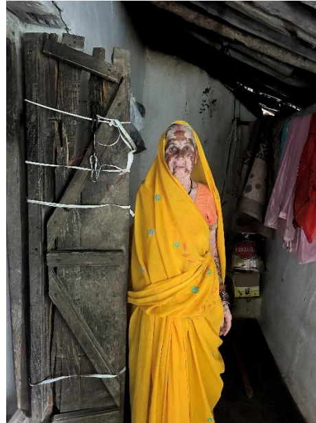
Damages caused to windows and door while sloth bear entering the Kitchen in Kokpur village
