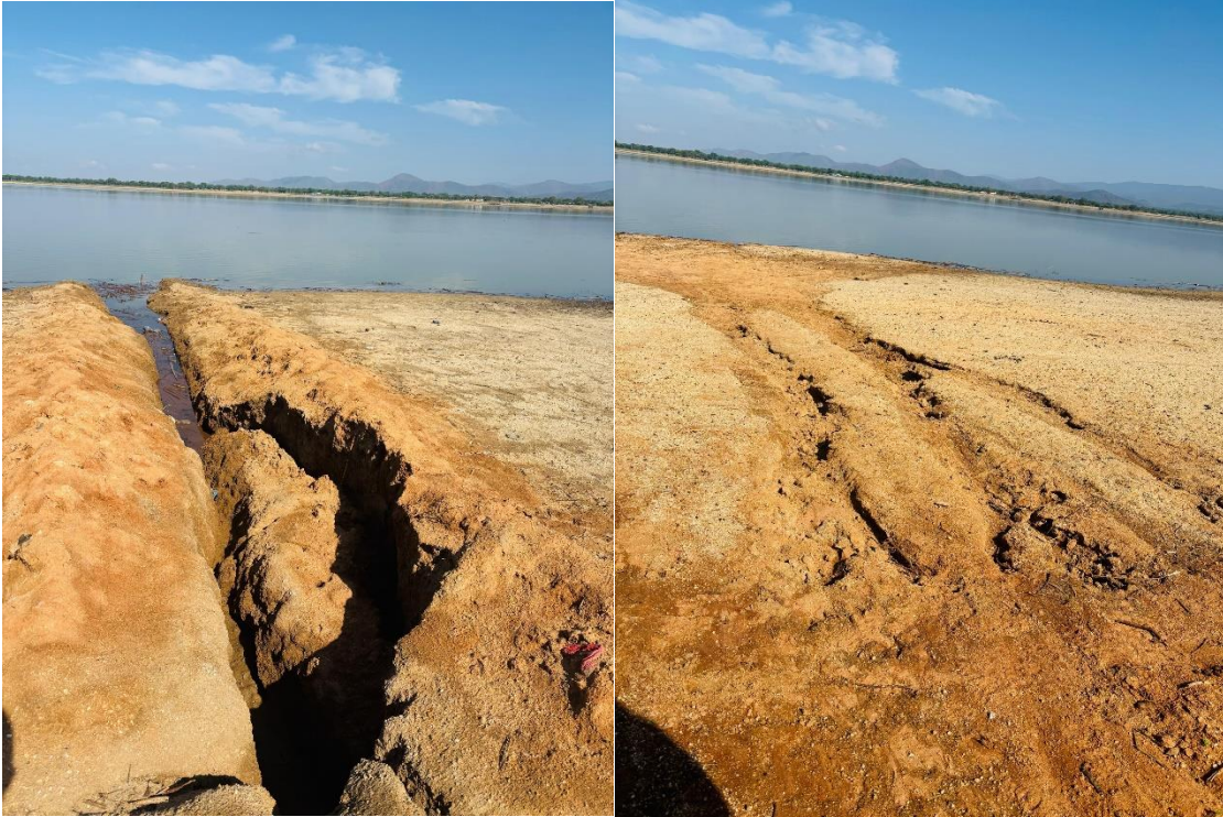
Figure 04: Unregulated construction of water channels used to extract water from the dam for agricultural purposes. Photo credit © Frank-UDOM, 2025.
